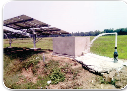
SPV Water Pumping Systems installed in village of Medinipur (West Bengal)
